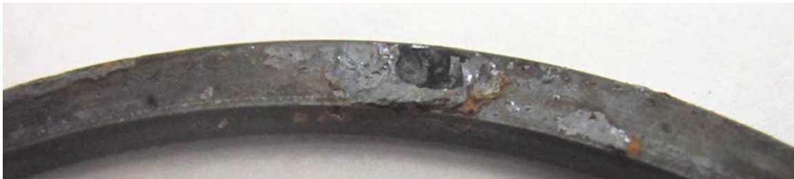
Figure 2: Close up of International Chemical 152 coated part to show corrosion
